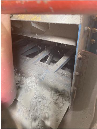
Collect excavated material at end of screen to ensure a more representative mixture
